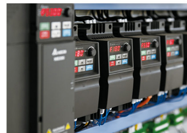
电气设备 Electrical equipment:
